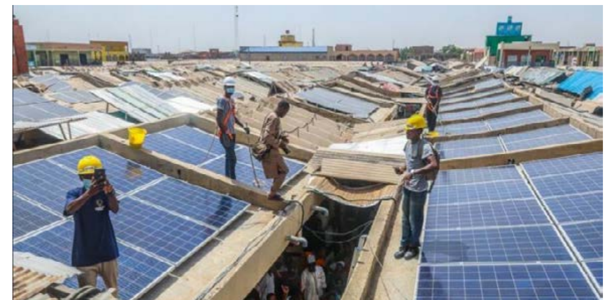
Solar panels on stalls of Sabon Gari Market, Nigeria
